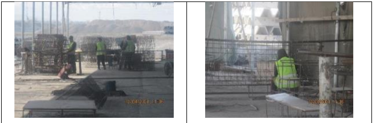
Figure 40 Production of reinforcing welded meshes, frames for the production of reinforced concrete structures
