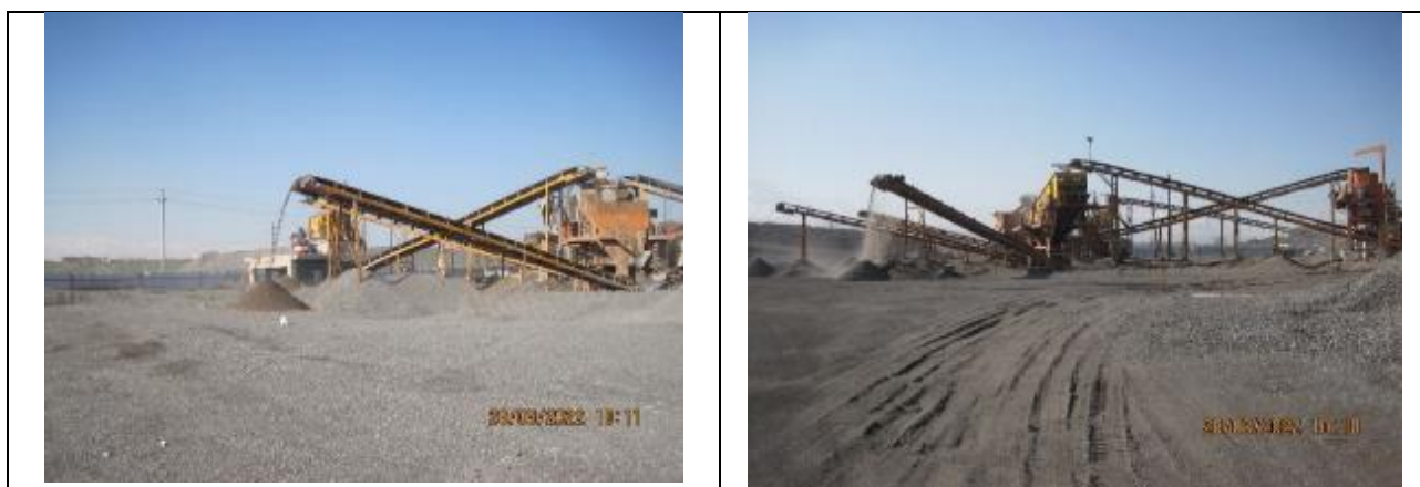
Figure 38 Operation of a stone crushing plant on moistened raw materials
