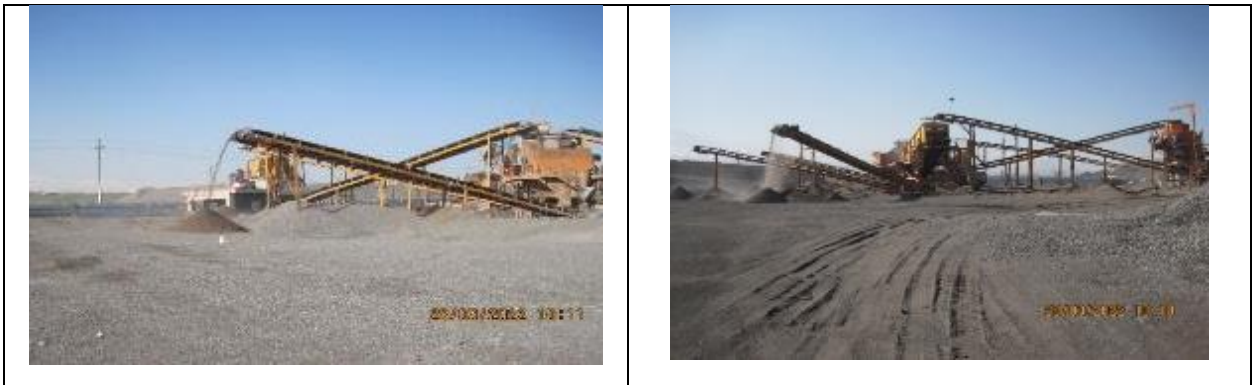
Figure 20 Stone crushing plant.
