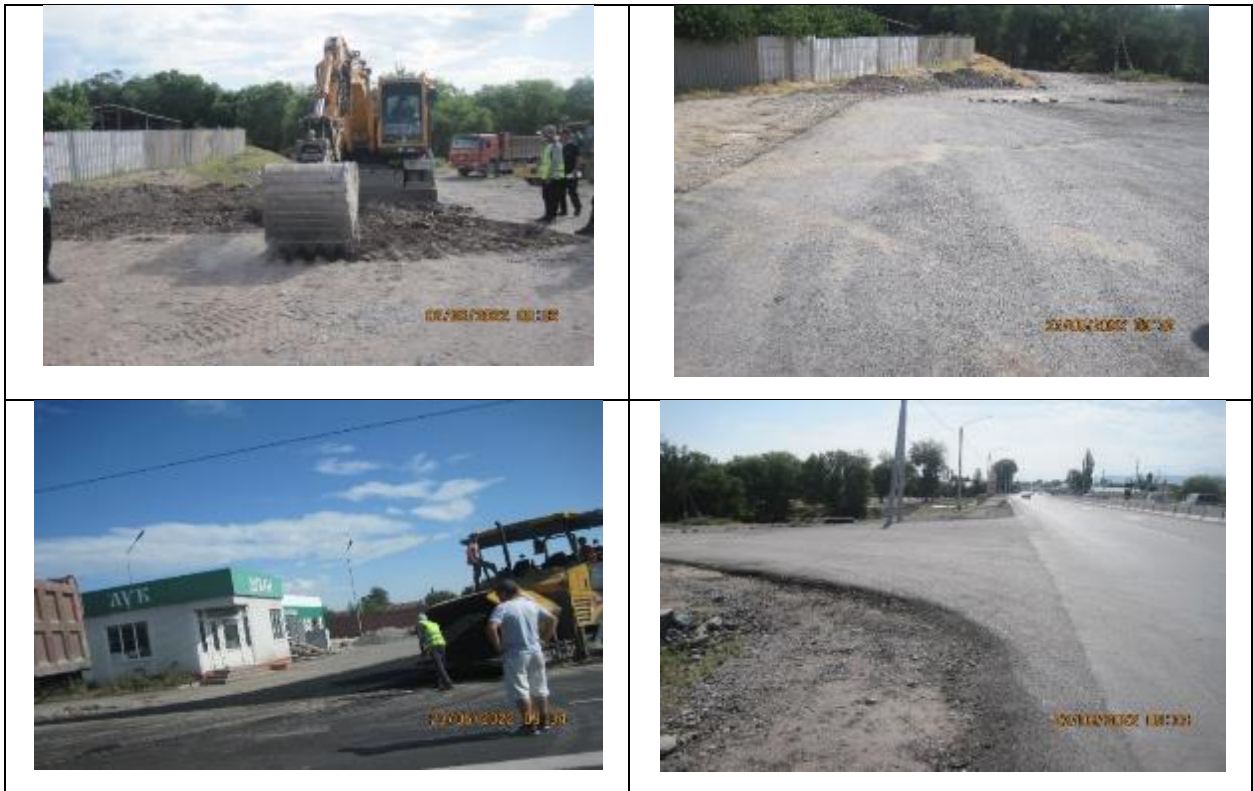
Figure 7 Laying asphalt at junctions to the streets adjacent to the road. Belovodskoe village
