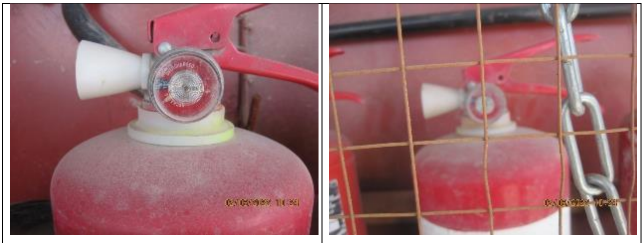
Figure 47 Fire extinguishers installed with violations on the territory of the production site.
