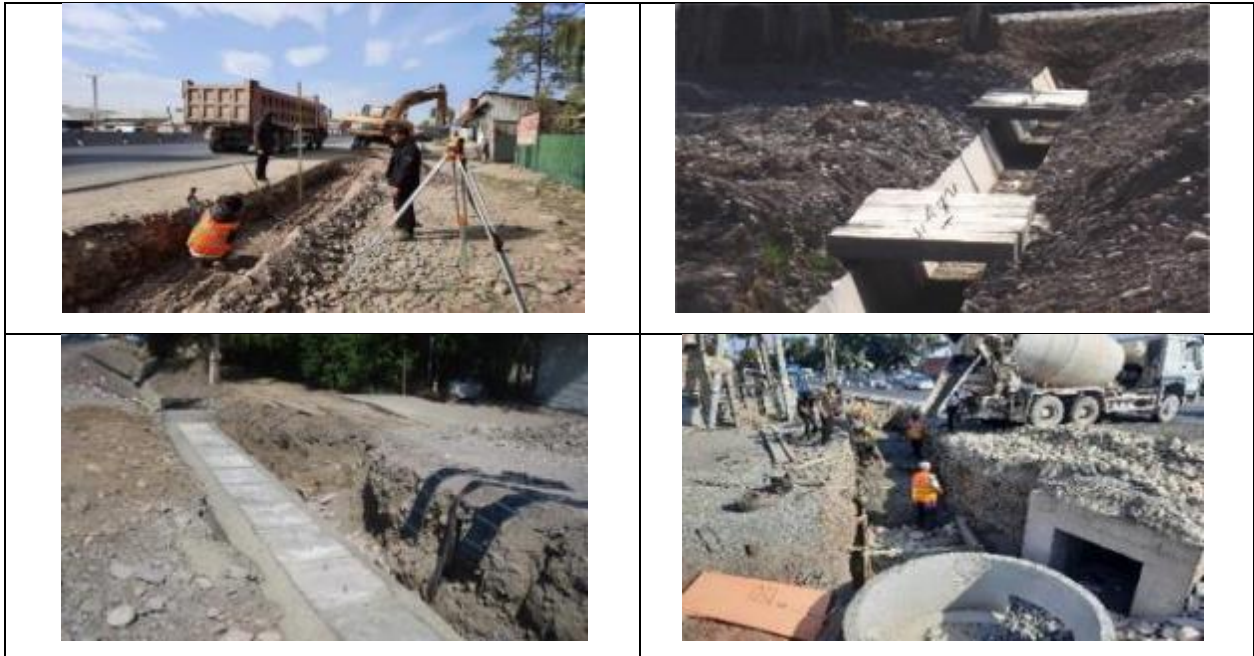
Figure 5 Installation of roadside culvert ditches and crossings to private houses and streets adjacent to the road
