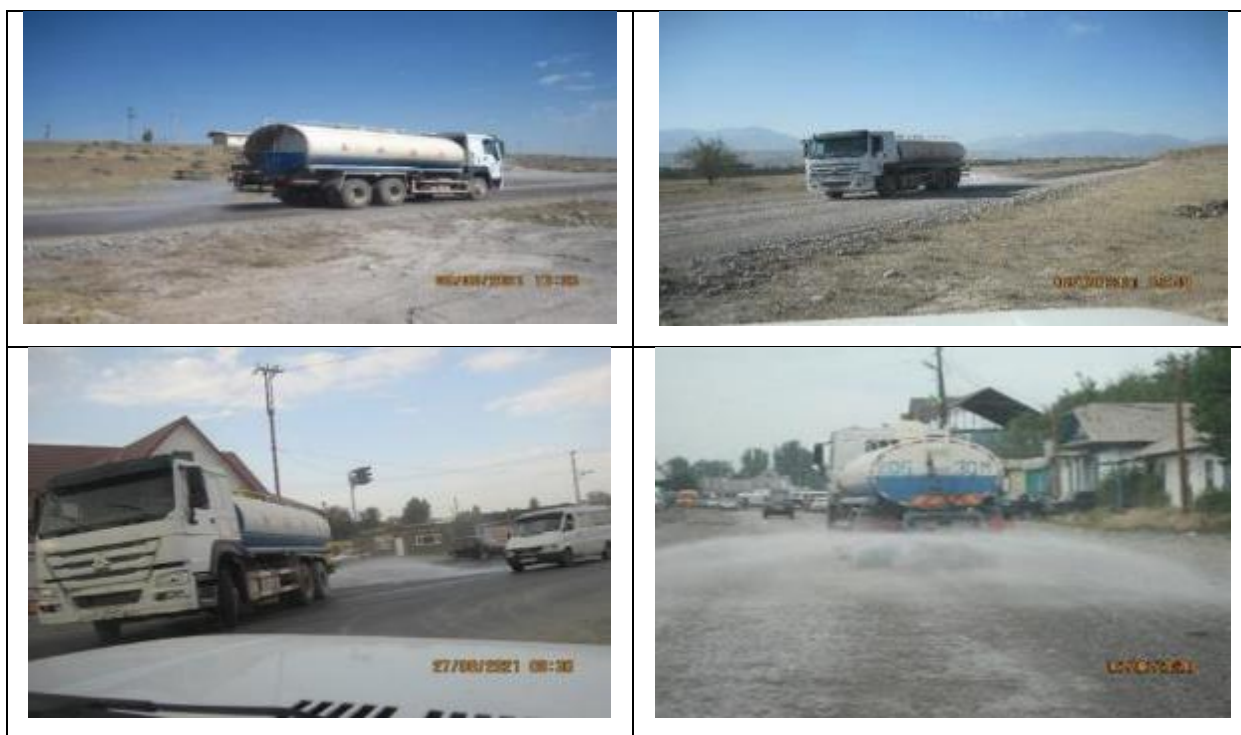
Figure 16 Dust suppression (water sprinkling). The road to the production site and at the road construction site
